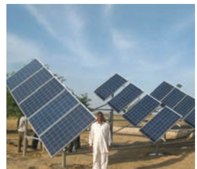
Solar Water Pump
