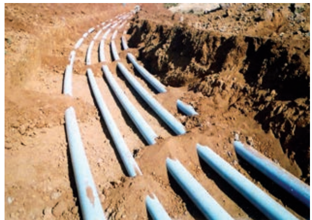
PVC Pipe for water supply
